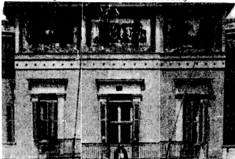
Fig. 7 Mosaic of the rectified images of the upper part of planes 2, 1 and 3 of the southern side (at scale 1:100)
