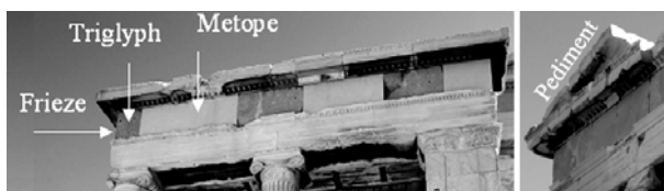
Figure 2. Missing architectural elements
