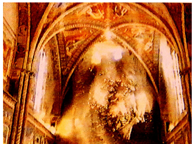
Figure 13. Collapse of the ceiling of the Assisi Basilica during the earthquake of 27 September 1997 [6]
