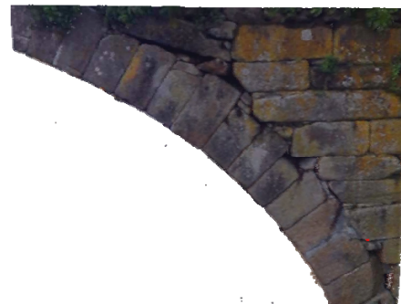
Figure 8. Coloured scan of a crack in an arch ring of Traba Bridge.
