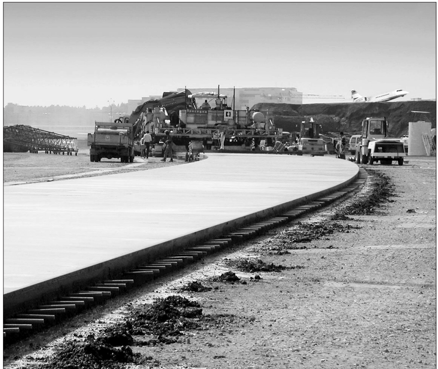
At Zurich Airport, where this interview took place with Hans Hess, a Leica Geosystems 3D machine guidance system is being used automatically to guide and control a slip-former for the construction of concrete run ways. These run ways have horizontal and vertical precision of respectively, one centimetre and three millimetres. The machine guidance system concerned consists of two Leica TCA 2002 total stations and a control unit directly fitted in the slip-former drivers' cab. (Source: Fritz Staudacher, Leica Geosystems).
