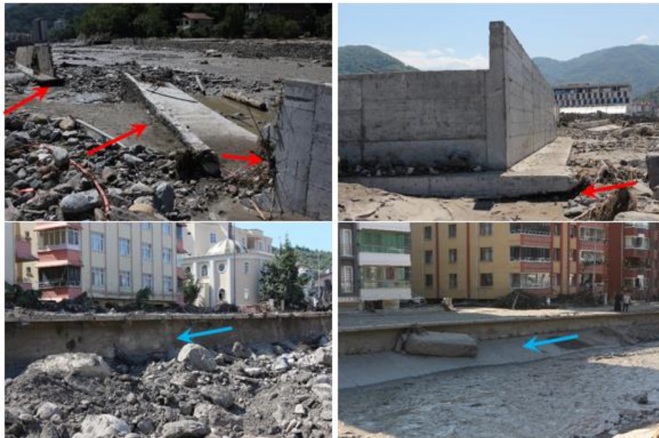
Figure 17. Damaged and intact retaining walls (Bozbey et al., 2022).
