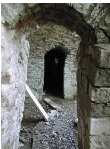
figure 5: deformation of the entrance in the closed casemate 9
