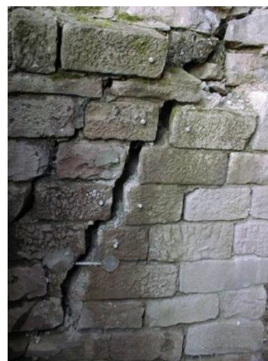
figure 6: crack in east casemate 7
