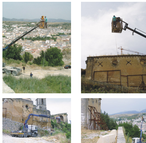
Figure 4. Stereopairs in the west walls were taken with the help of a mobile hoist.
