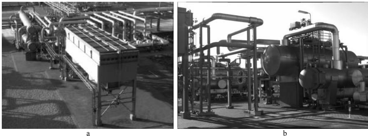
Figure 4. Images of the gas-drying unit.
