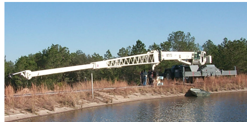
Figure 2. Crane used to position thermal camera over float
