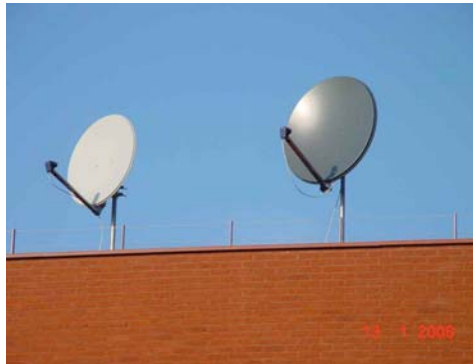
Figure 1. EUMETCast reception antenna at VITO (left) and DDS reception antenna (right)
