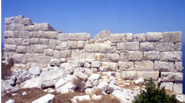
Figure 3. Photograph of the east facade before the collapse of the northeast corner (KB' EPKA)
