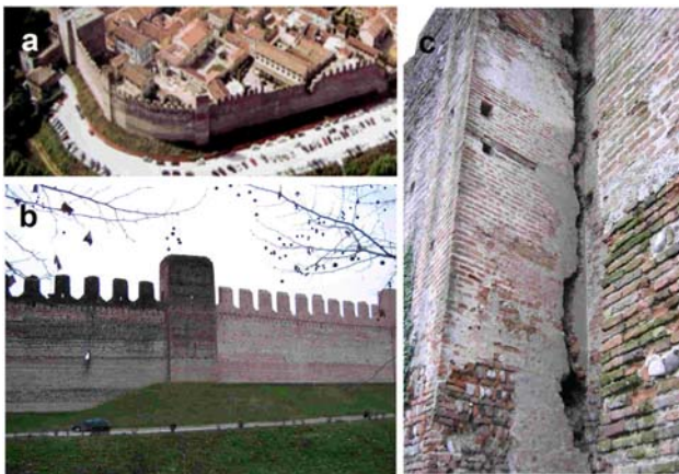
Figure 2. a), b) Different view of the analyzed area; c) Structural degradation of the town-walls
