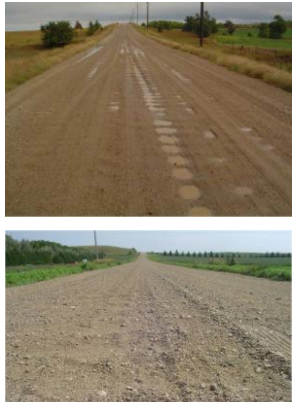
Figure 2. Ground images of deteriorated unpaved roads. Above: Serious distress with potholes and bad surface drainage. Below: Loose aggregate with corrugation.
