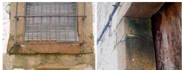
Figure 8. Deterioration of stonework in various cases.
