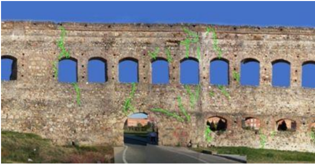
Figure 9. Some of the cracks detected in the Aqueduct of San Lázaro.
