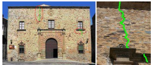
Figure 6. Cracks in the Episcopal Palace.
