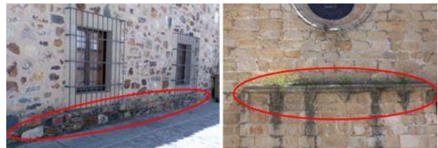
Figure 7. Damp in the Palace of Diputación and the Church of Santa María.
