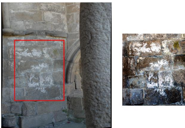
Figure 1. (left) Image of the damaged chosen chapel, taken with a digital camera; (right) 2D image of the selected region obtained from the 3D information of the colored point cloud.
