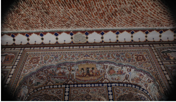
Mohrakashi work: Scratched ceiling
