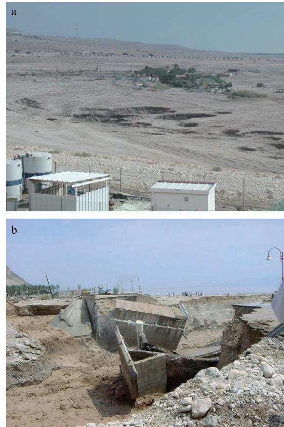
Figure 1. a) Collapse sinkhole field near a beach resort, b) collapse of a bridge following a flood as a result of a headcut backward migration along the stream channel.
